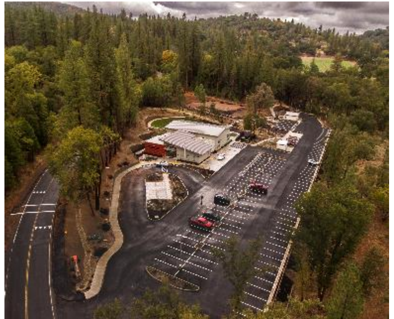
Shown above is the final stage of construction on the Tuolumne County Resilience Center at Groveland. The 5.5-acre site includes a community event center, ample parking, an outdoor grass amphitheater, a standalone exterior restroom, and an ADA compliant nature trail equipped with picnic tables, benches, a bridge, and watering stations.
